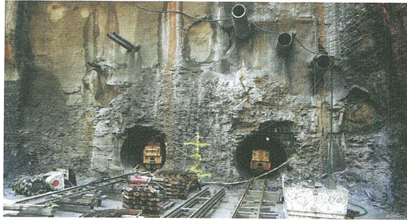
An arch of seven interlocking TBM-bored cover tunnels was used at the Billy Bishop pedestrian tunnel, Toronto
